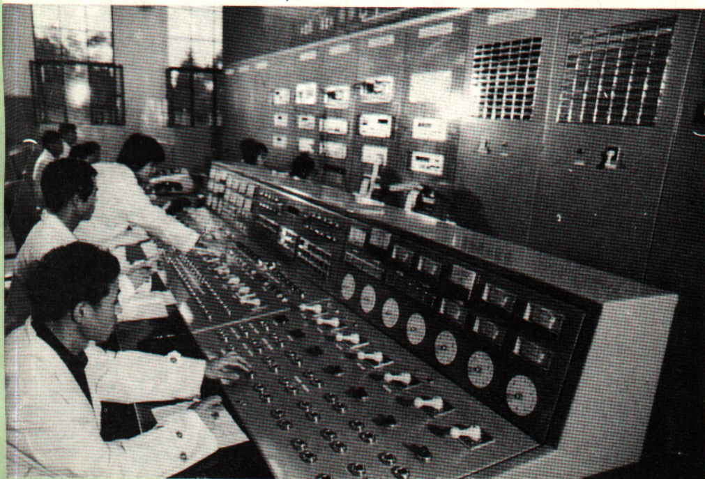
The central control room.
