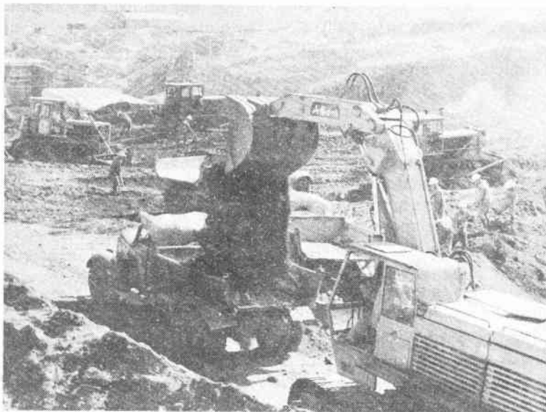
A worksite of the project to lead the Luanhe River waters to Tianjin.
