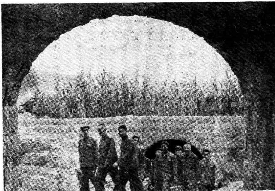
Delegates to the recent national conference on learning from Tachai visiting the Shihping culverts.
