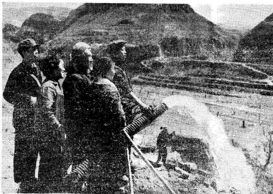
An electric pumping station, equipped with county-made motors and pumps, irrigates the land.
