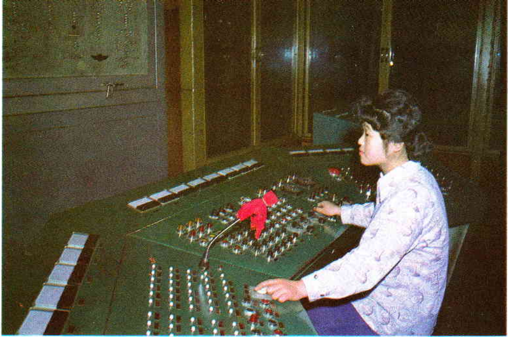
Control room for a foundry shop.
