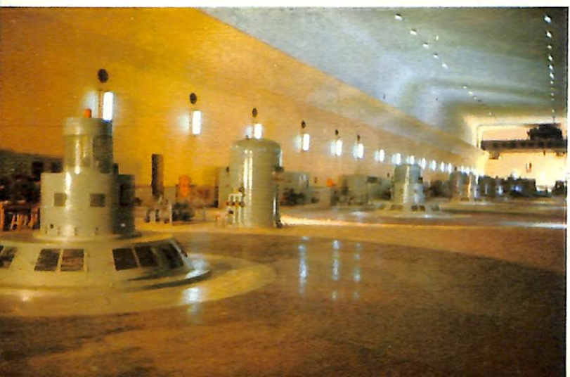
The China-made 150,000-kilowatt generator sets.
