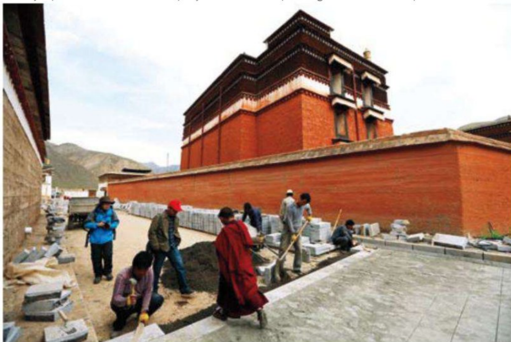
A major part of the renovation project involves improving infrastructure. by Wan Quan
