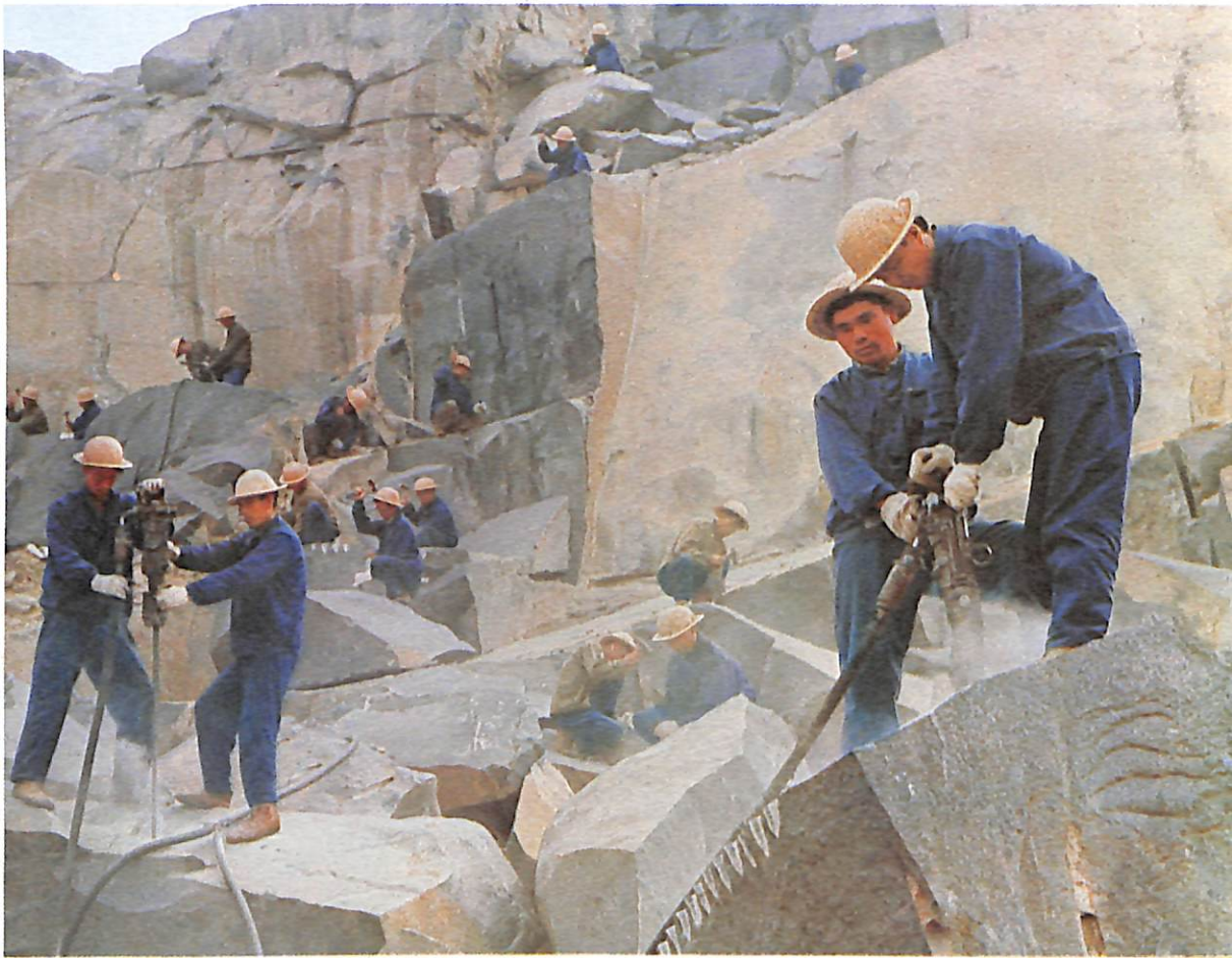
Workers at the Tsinan Quarry, Shantung Province, cutting and processing granite slabs for facing the podium.
