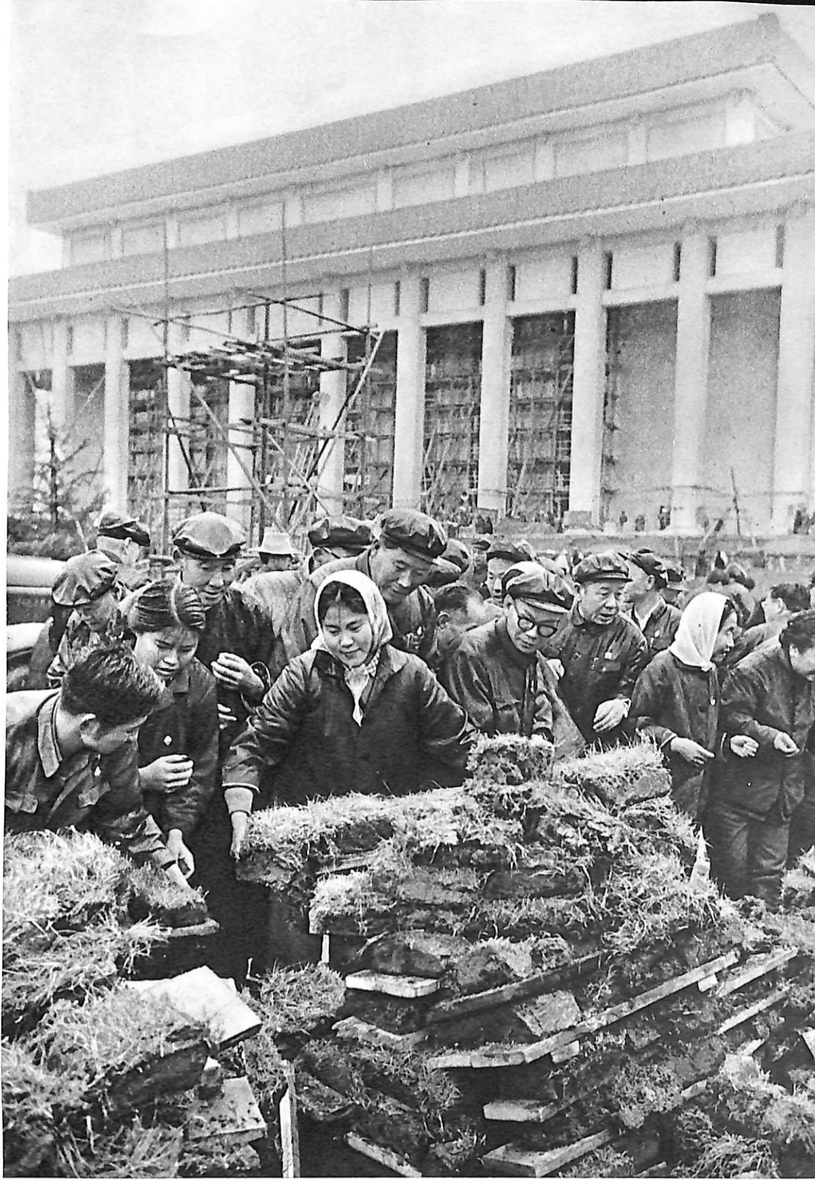
In the name of China's working class, representatives to the National Learn-from-Taching Conference taking part in voluntary labour at the construction site.
