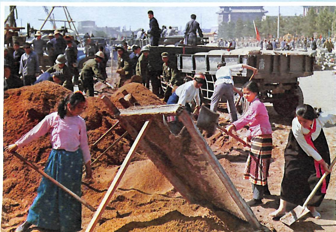
People of various nationalities from all parts of the country taking turns in voluntary labour at the construction site.
