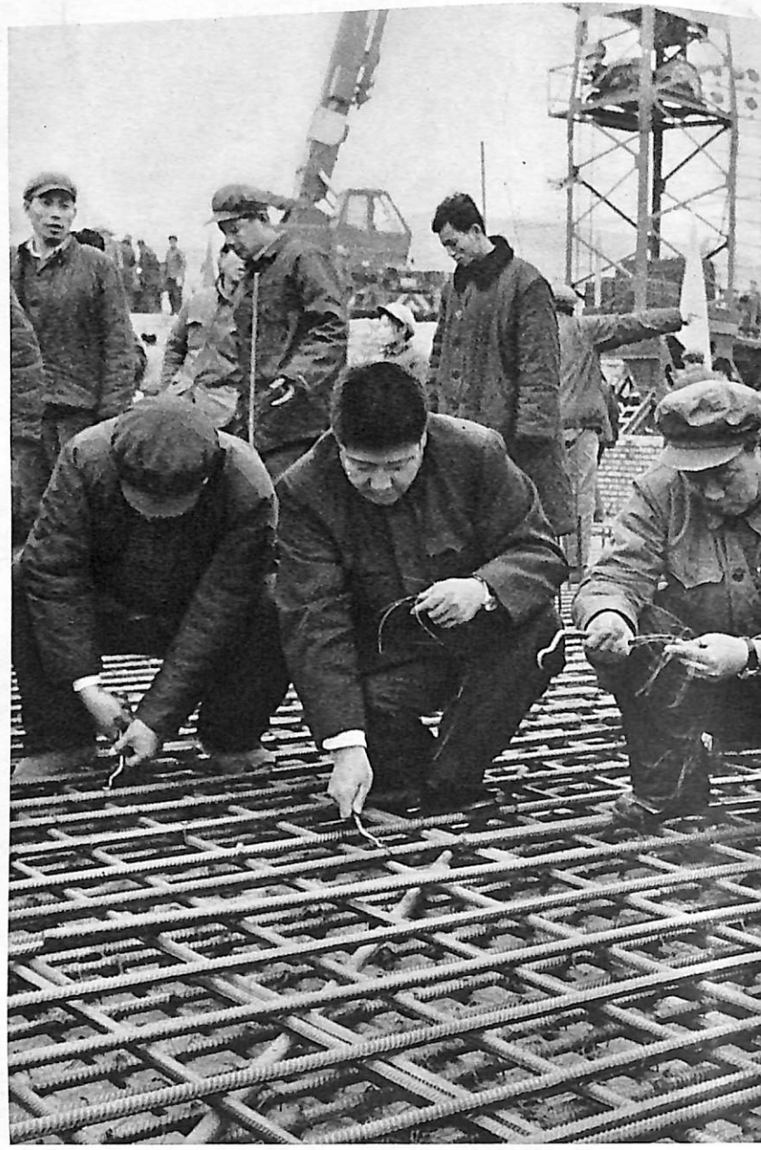
In the name of hundreds of millions of peasants, representatives to the 2nd National Learn-from-Tachai Conference taking part in voluntary labour at the construction site.
