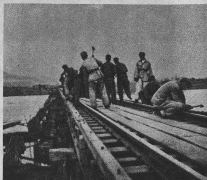
No matter how difficult the circumstances, the railway corps of the Chinese volunteers carry out immediate repairs on bomb-damaged railways.
