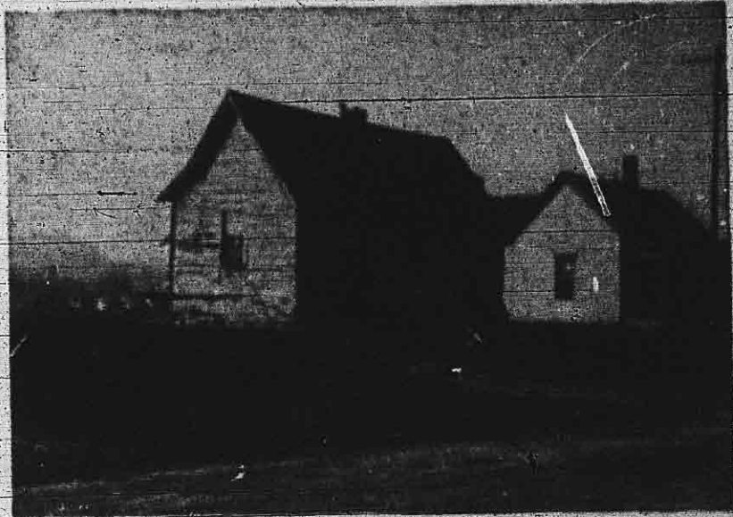
Company owned houses in Elizabethton, Tenn. where rayon workers are forced to live. Though rents are high in comparison with wages the workers receive, the company refuses to make repairs on the houses.
