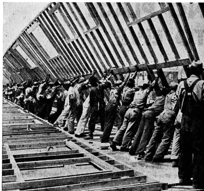
Palmer, OWI Raising the frame of a four-unit war workers' home at Erie, Pa.—
