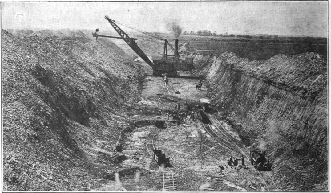
LOOKING DOWN ONE OF THE LATERALS FROM THE TOP OF ONE OF THE EARTH PILES. The part beyond the shovel has been worked out from the other end.
