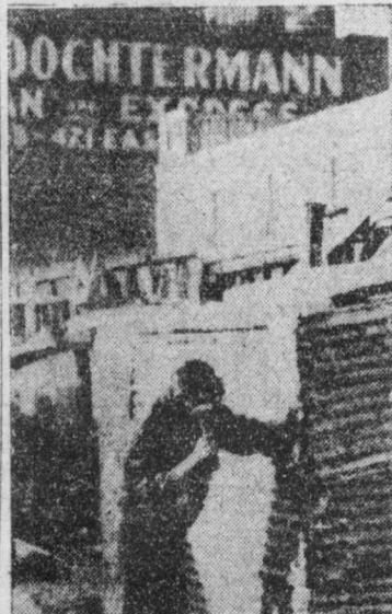
Unemployed and homeless, these men are building a shack for the fourth winter of cold and hunger. There are 70 more shacks like this at East 10th St. along the East River. Many were built by men who put up, just before the crisis, some of the big skyscrapers they can see from their present hovels.
