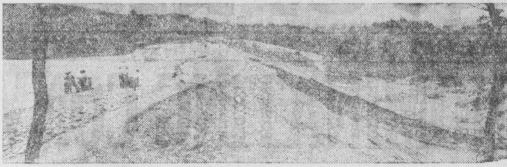
Rifts in the earth dam across the Saluda River at Table Rock, S. C., are shown at picture on left. The dam threatens bursting to engulf thousands of poor workers and farmers, repeating the San Francisquito dam tragedy in California. Photo at right shows workers struggling above the roaring waters of the South Saluda River in an attempt to open a valve and relieve pressure of the flood.
