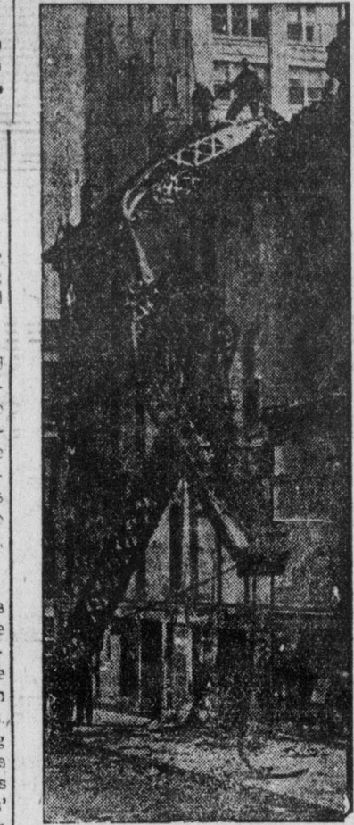
Twenty-four floors above the street, a ten-ton girder suddenly plunged downward, carrying a 95-foot steel boom with it, when the boom gave way on site of a new 56-story building. A large number of workers below and many pedestrians narrowly escaped death as a result of the crash.
