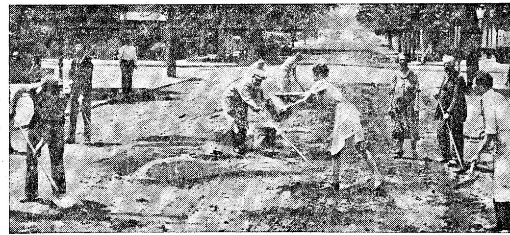
While the Tammany bandwagon rides merrily along a pathway of graft to the democratic convention at Houston, residents of Brooklyn streets are compelled to resort to temporary makeshift measures to make streets passable to vehicles and pedestrians. Above, residents tired of being ignored by Tammany repairing the street.
