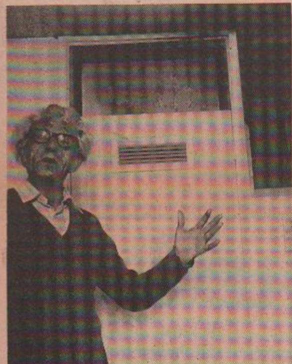
Robert Ayres, who lives with his wife Margaret in one of the pensioners' houses on the estate. The central heating boiler just caught fire. It is encased in a cupboard. The Fire Inspector said the systems were dangerous. Now the GLC have switched them off in all the old people's flats. Lucky the weather is warm.
