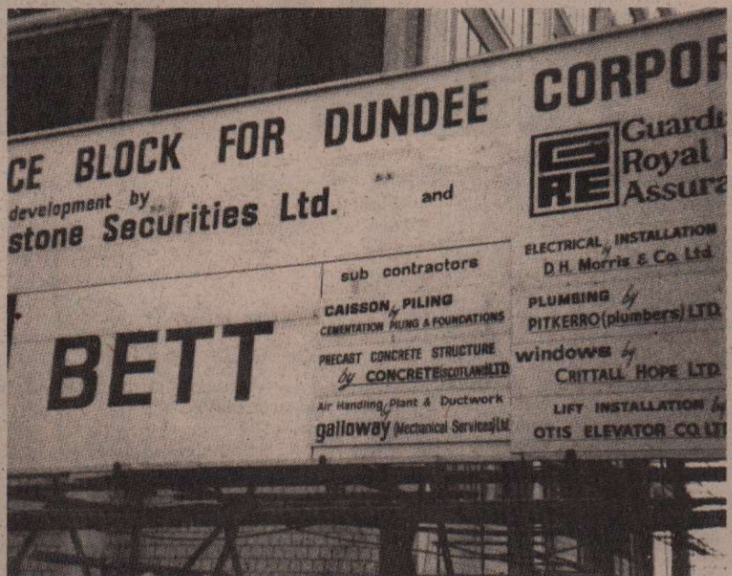
The new Tayside region HQ: note the name of Galloway, a firm owned by Councillor Harry Dickson
