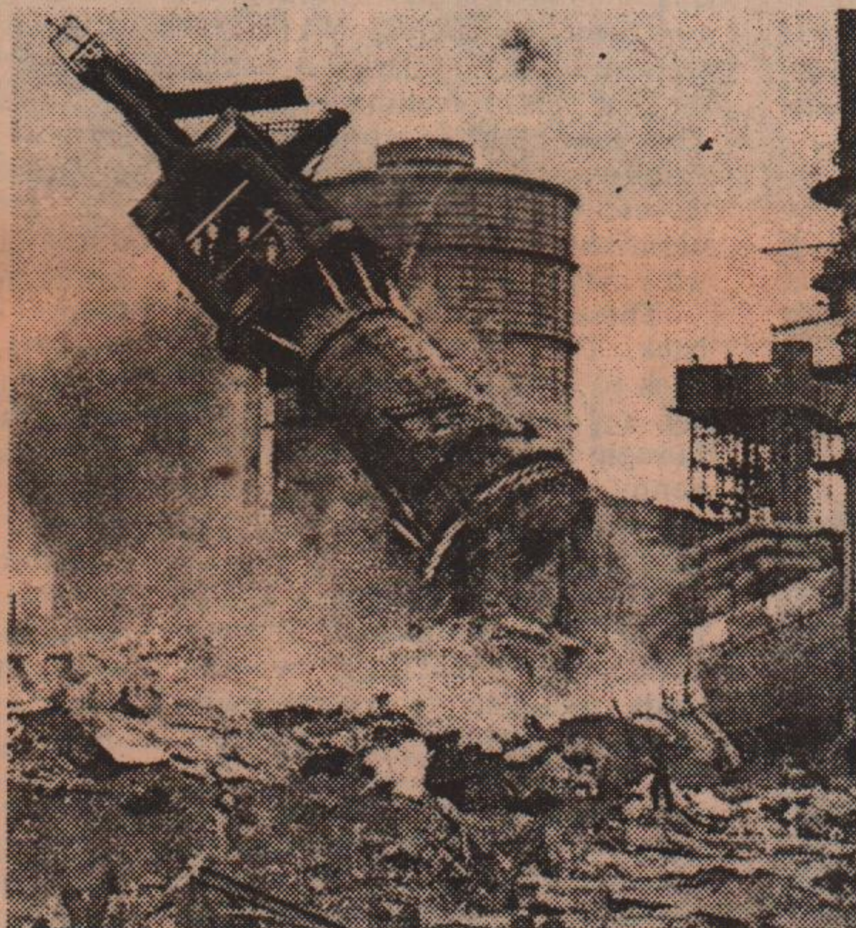
Flashback to the demolition—a year ago—of the blast furnace the British Steel chairman said might be brought back into operation.
