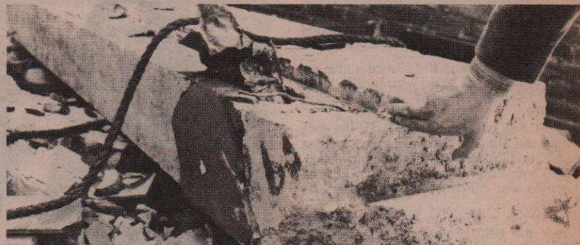
A section of the perimeter beam at Camden shows the narrow ledge—only 40mm wide—which supported either end of the roof beams.
