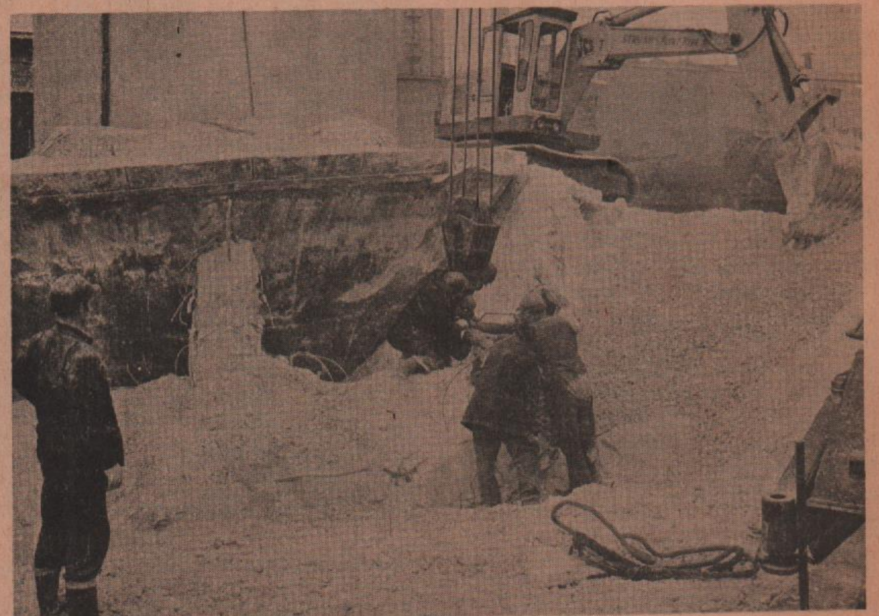
Workers digging desperately for the missing men after the silo collapse
