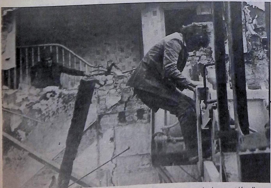
The work is dangerous. The workers dodge falling bricks and timbers as the bulldozer pushes down an outside wall, or as the crane driver guides the concrete ball that swings from his crane to topple stronger buildings.
