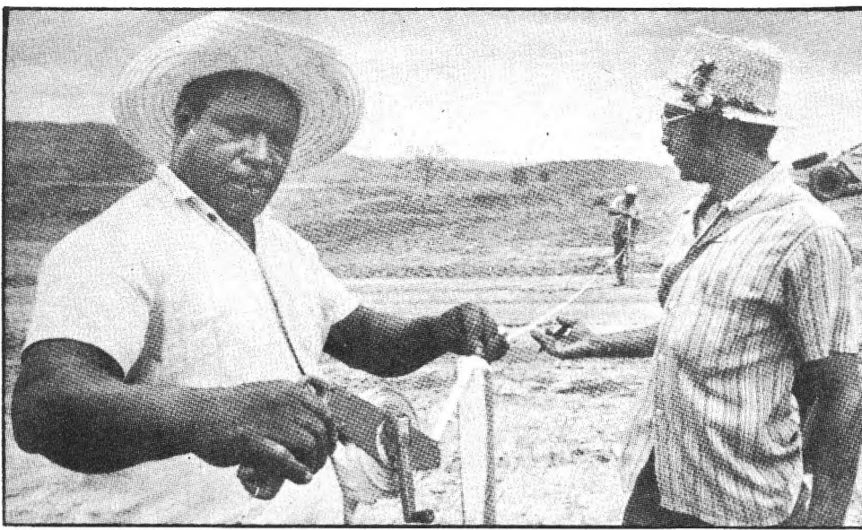
CUBAN "AID" in this construction project is part of increasing Soviet-Cuban presence.
